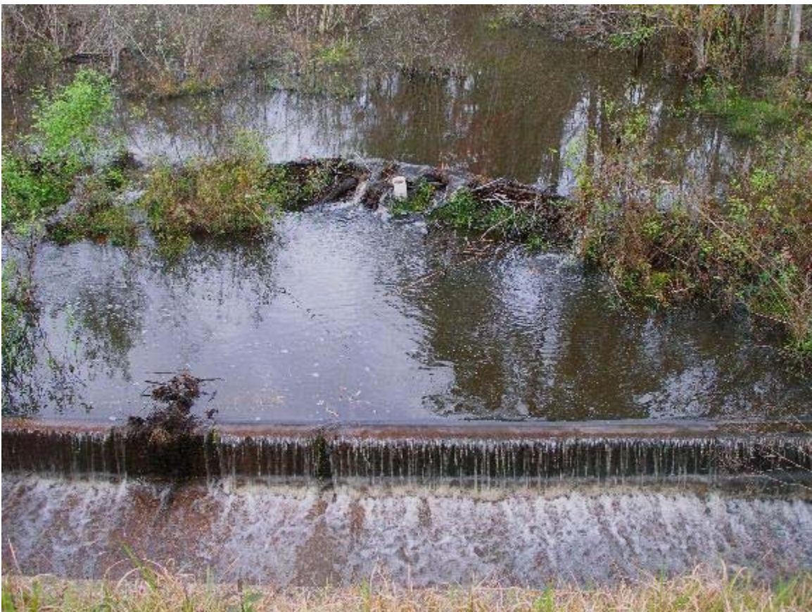
Figure 65 Upstream portion of sampling site CB1 featuring a cement overflow wall and beaver damming
