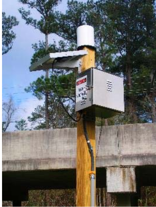
Figure 25 Continuous real-time monitoring station installed at site CB5
